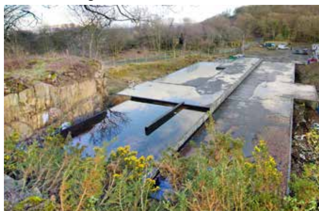
SOC is watertight with the new roof covering. Here you can see the standing water on top of the building. This picture also shows the extensive felling which we've done and the clearance of the car park at the top right of the picture
